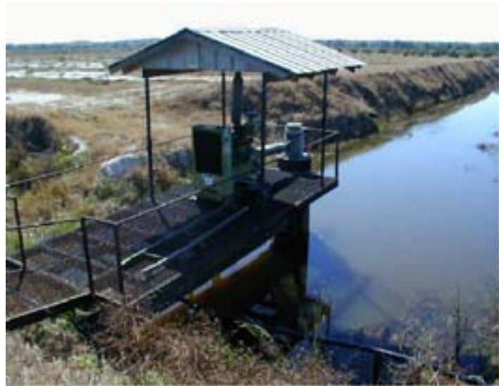
Figure 12. Drainage pump station in citrus grove.
