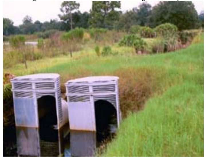
Figure 15. Water control structure used to maintain water level and drainage rate from citrus grove.
