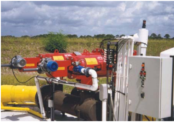
Figure 7. Control panel for automatically backflushing filters based on pressure differential between inlet and outlet of filter.
