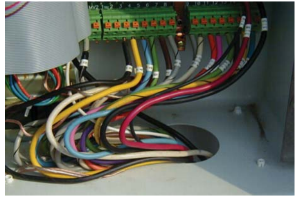
Figure 4. Multi-colored low-voltage wiring used to connect controller to valves and other control devices.
