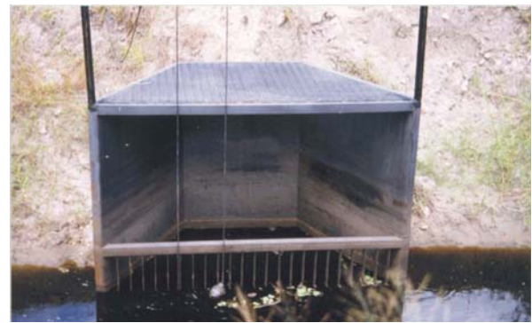
Figure 9. Float controls for drainage pump.
