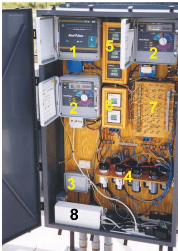
Figure 14. In-field controls for a centrally-controlled citrus irrigation system including: 1) on-site communication, data storage, and control device; 2) valve, pump, and accessory controllers; 3) phone connection; 4) sensor decoders; 5) flow monitors; 6) pressure and water level monitors; 7) manual over-rides; 8) power conditioning and surge protection.
