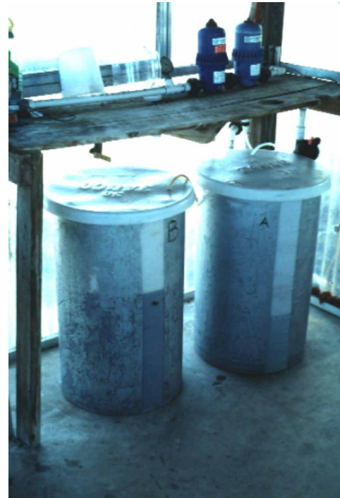
Figure 2. Stock tanks containing concentrated fertilizer are located under the fertilizer proportioner bench to conserve space.
