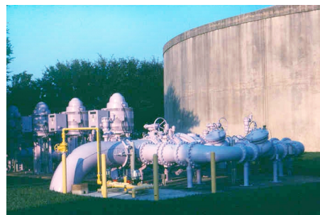
Figure 1. Purple pipes identify reclaimed-water transmission. Credits: Tom Yeager
