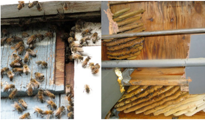
Figure 13. Nuisance colonies of European honey bees, Apis mellifera Linnaeus. Left: worker honey bees at the entrance of a colony in the exterior wall of a house. Right: the underside of a carport roof has been cut away to expose the wax combs of a colony.
