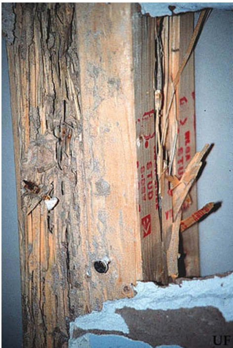
Figure 10. Damage and fecal spotting by Heterotermes subterranean termites in dry framing, Miami, Florida.
