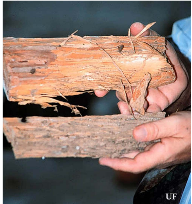
Figure 11. Heterotermes subterranean termite damage showing dry and shredded appearance of wood, Miami, Florida. Credits: Rudolf H. Scheffrahn, University of Florida
