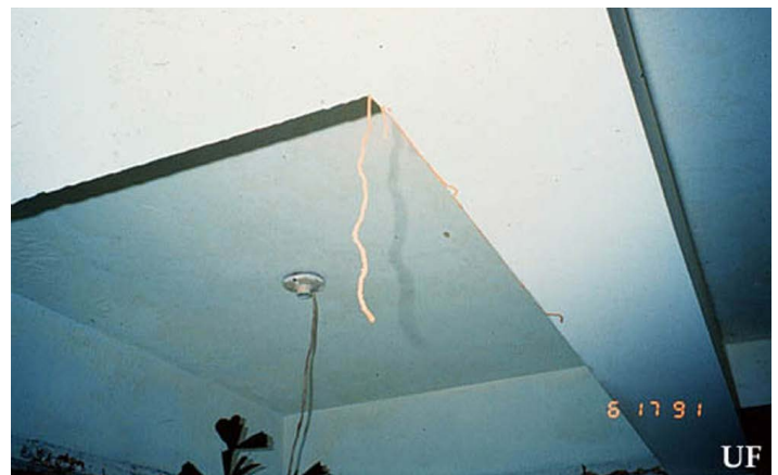
Figure 12. Heterotermes subterranean termite foraging tube dropping from living room ceiling, Santo Domingo, Dominican Republic. Credits: Rudolf H. Scheffrahn, University of Florida
