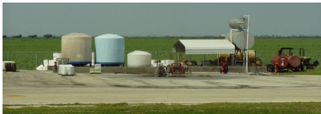
Figure 6. A Permanently Installed Containment Area for Large Quantities of Pesticides Credits: UF/IFAS Pesticide Information Office
