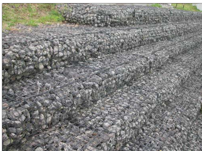
Figure 6. Use of gabions for stabilization of a canal side-bank. While expensive, these materials effectively prevent erosion in canal/ditch areas subject to high flow velocities. Credits: BJB
