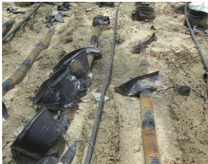
Figure 2. Polypropylene ground cloth was stripped away from this pot-in-pot production area by wind and water during Hurricane Matthew in 2016.
