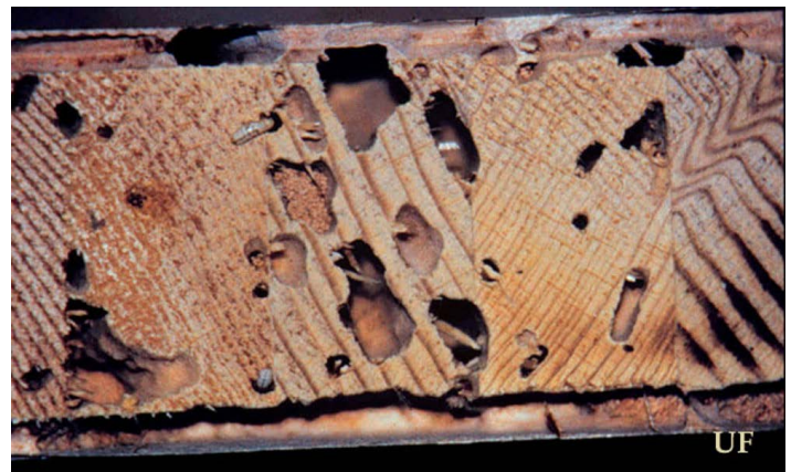
Figure 7. Damage (wooden door) caused by the West Indian drywood termite, Cryptotermes brevis (Walker).
