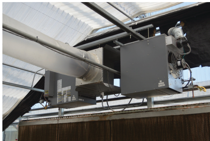
Figure 3. Fan-jet poly-tube system with heaters.
