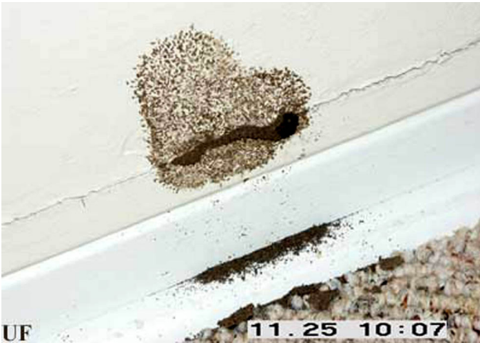
Figure 6. Prorhinotermes simplex (Hagen) termite flight tube emerging from interior wall above molding. Credits: Rudolf H. Scheffrahn, UF/IFAS
