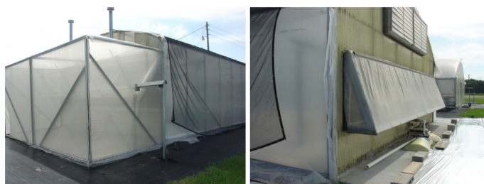
Figure 2. Insect screen covering air intake area.
