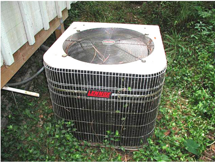
Figure 10. A typical AC unit attached to a house. Credits: Mark E. Hostetler, 2006.
