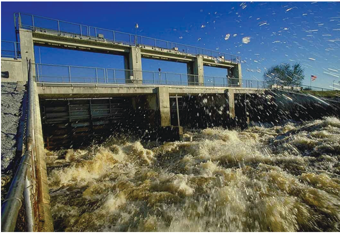
Figure 11. Water management structure releasing water (SFWMD)
