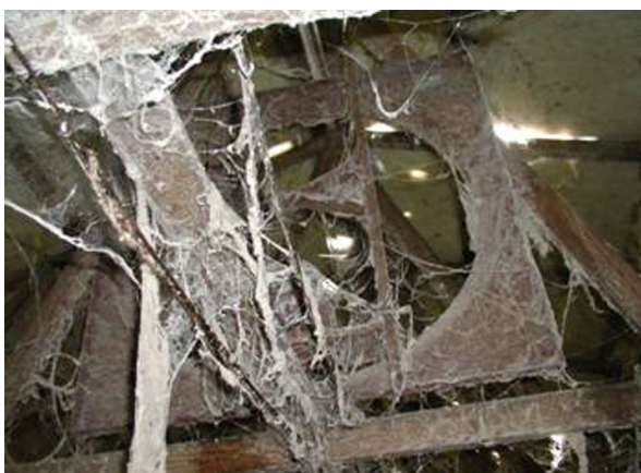
Figure 3. Broken fans and buildup of dust.
